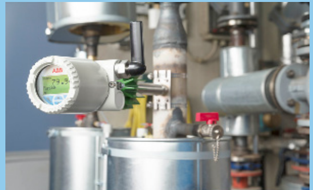
Installation of Sensors and meters to cover gaps in data required to produce PUE Calculations
